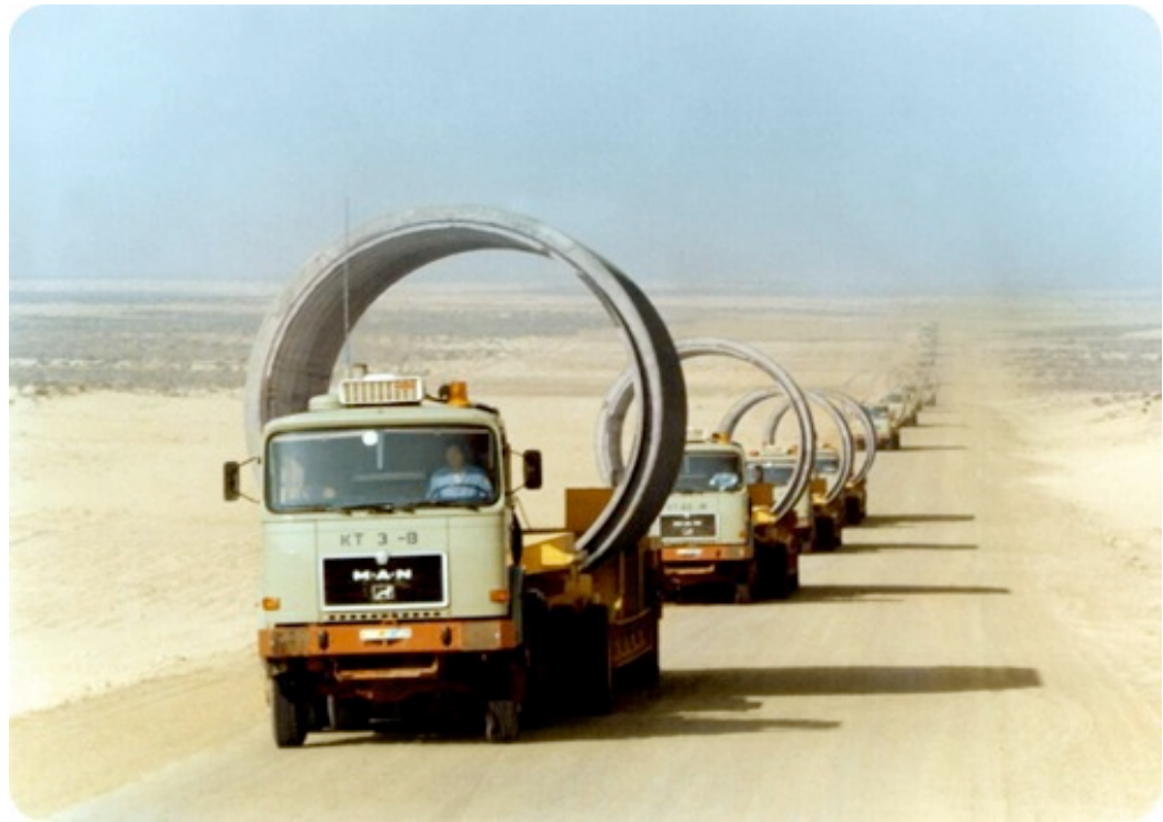
Figure 2: GMMRP pipe modules (4 metres in diameter) being transported to an installation site (Image: Galen Frysinger)
