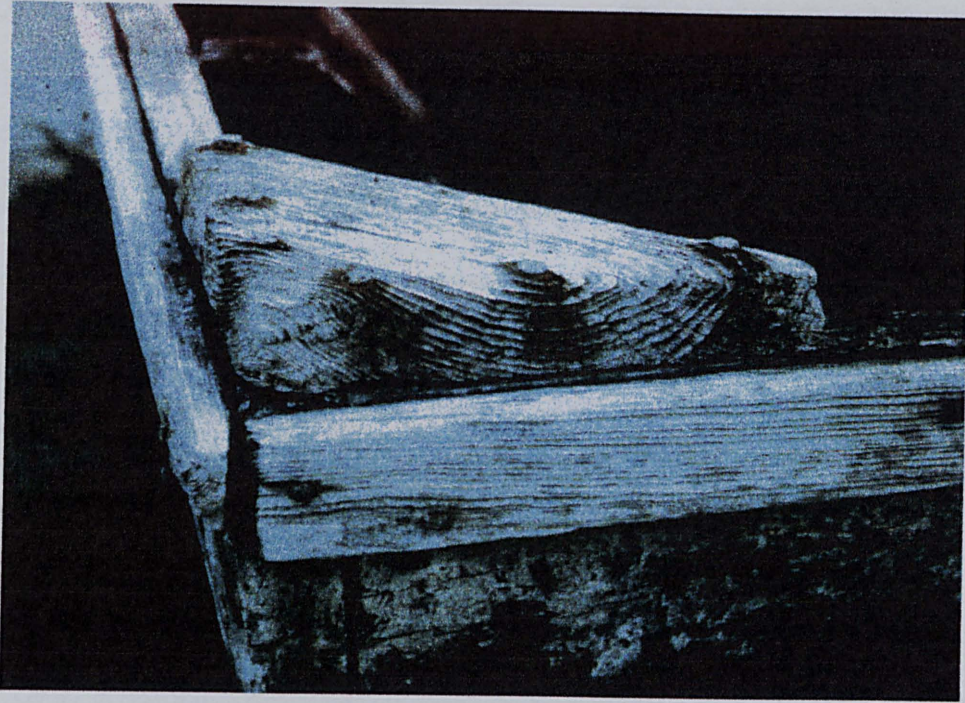
Figure 55: Photograph of large wire nails used to fasten corner fillets (photo: Mark Newell).
