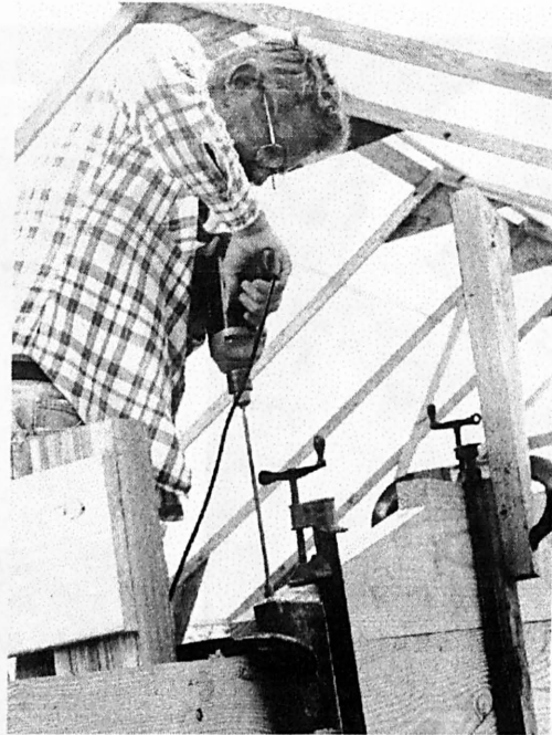
Figure 70: Power augur being used to drill holes for drift pins (photo: Mark Newell).
