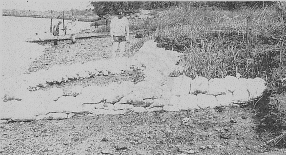
Figure 60: Exposed sections of the vessel are sandbagged by author (foreground) and USC staff (photo: Carl Naylor).
