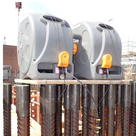
Figure 3.3. Fibre optic cable reels at one of the monitored walls, before they were integrated into the jumpform rig.
