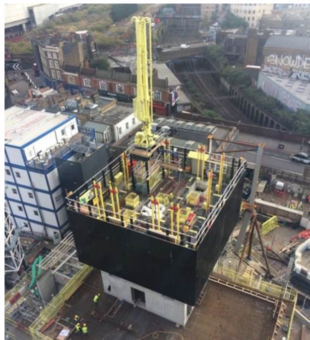
Figure 2.3. The lower levels of the core being constructed using an automated jumpform.
