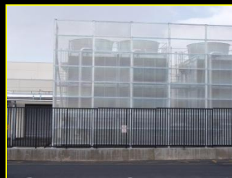
Compare LANL Q supercomputer's cooling towers
