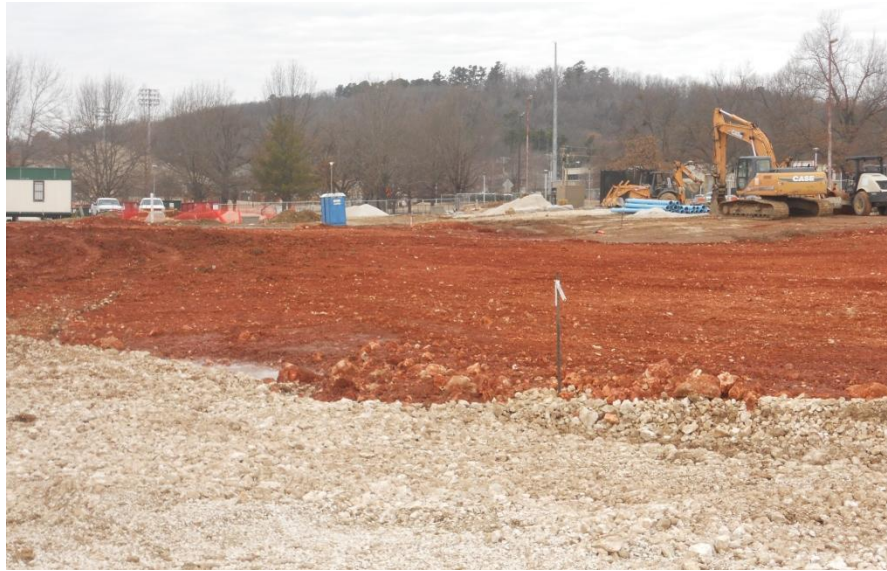
Figure 4.14. Example of a construction site near the Lot 56B infiltration sampling site. Topsoil has been removed and non-native soils have been introduced to the site and compacted.
