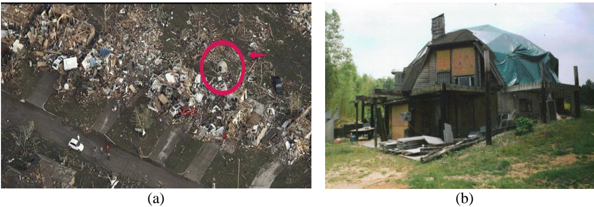
Figure 1.2: Dome survived with partial failure in (a) Moore, OK (Parker, 2011) and (b) West Jefferson County, NC (AGE dome, 2015)
