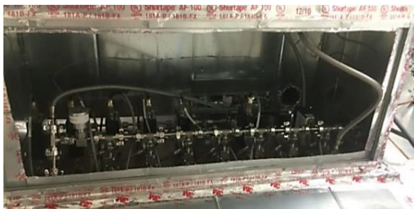
Figure 13. Secondary containment located above the gas manifold. All the MFCs and VCR connections were exhausted with secondary containment.
