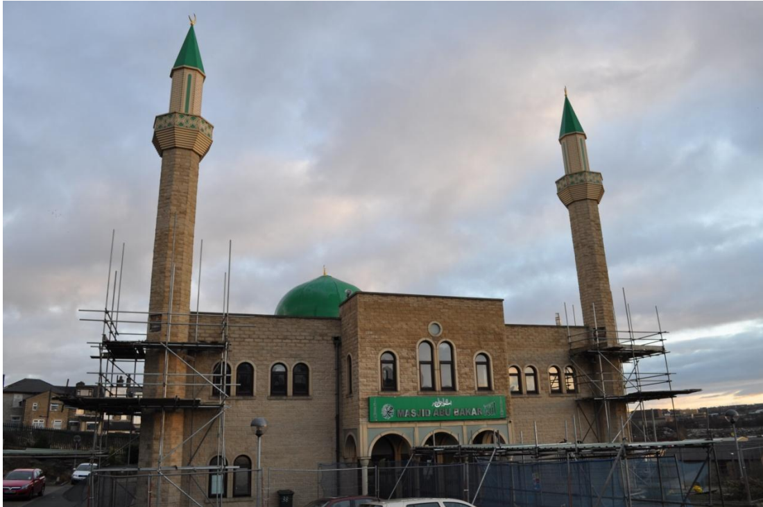
Picture 3-1: Surveys were conducted at the Abu Bakr Mosque on Steadman Terrace Road (Reid, 2010)
