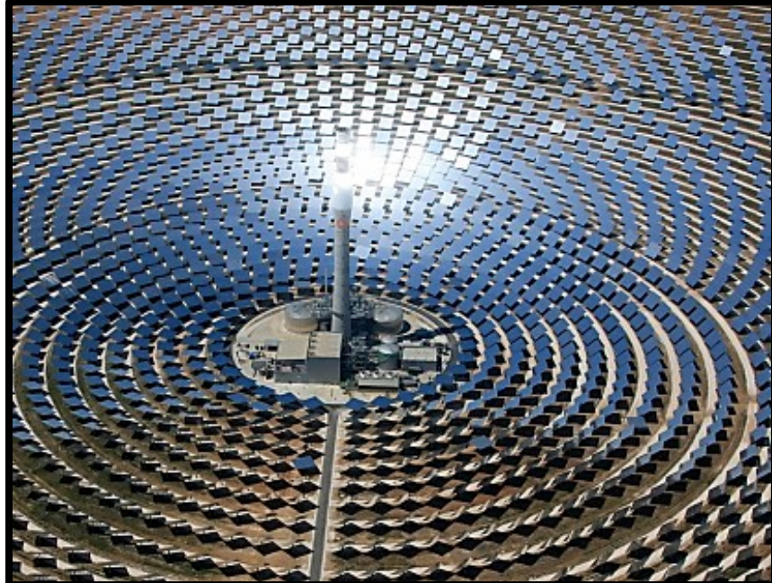
Figure 18: Central Receiver and Energy Storage Tanks at 19.9 MW Gemasolar Plant in Seville, Spain (Harrington, 2012)
