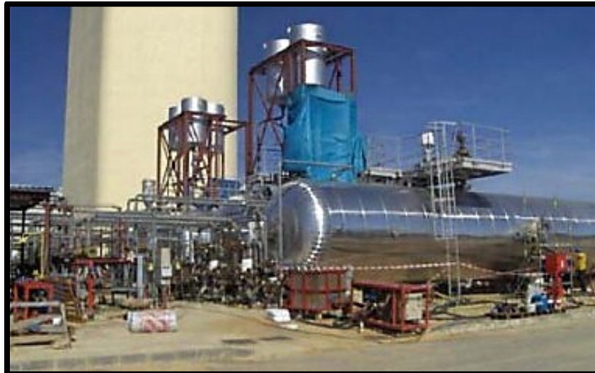
Figure 15: Energy Storage Tank at 10 MW Central Receiver ADS Plant in Seville, Spain (Medrano et al., 2010)
