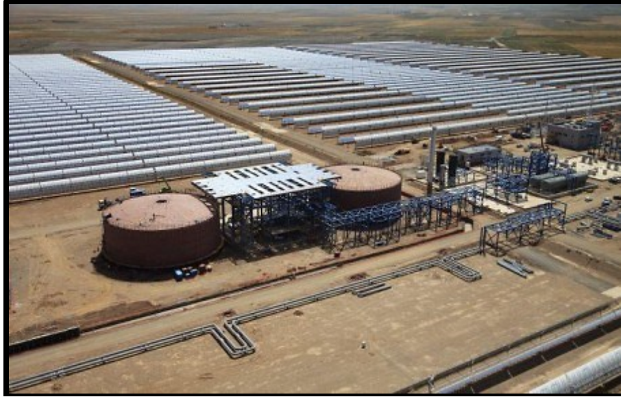
Figure 20: Two-Tank TES and Trough Array at 50 MW Andasol I in Granada, Spain (Craig, 2011)
