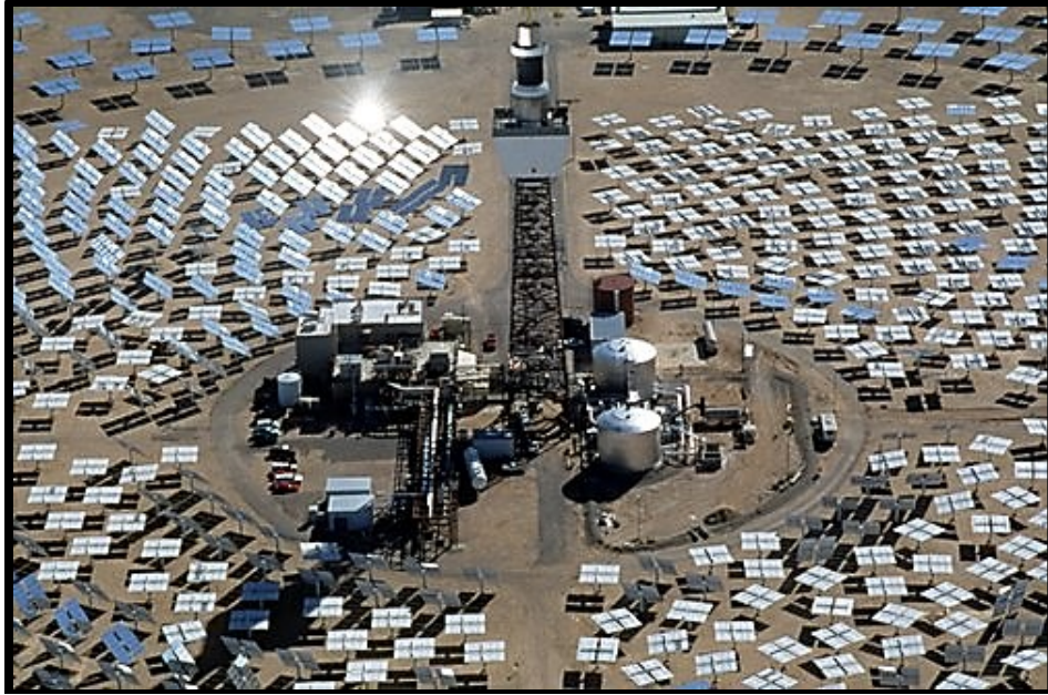
Figure 17: Central Receiver and Hot and Cold HTF Tanks at Solar Two in California (NASS, 2012)
