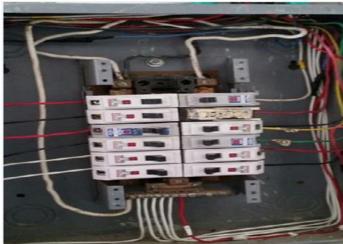
Figura 7. Barrajes tablero principal
