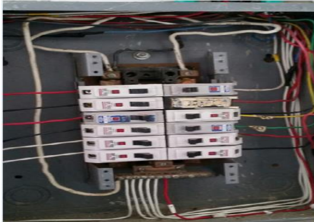
Figura 9. Barrajes tablero principal
