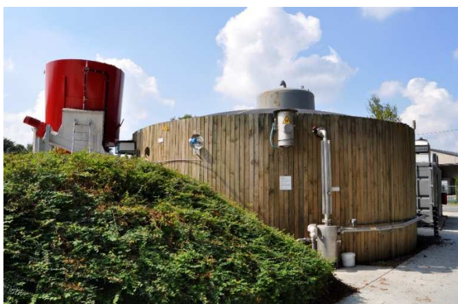
Figure 1: small-scale anaerobic digester
