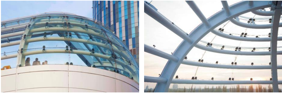
FIGURE 2.17: FLOREASCA CITY CENTER, BUCHAREST, ADHESIVE PRODUCER: SIKA NV (PHOTOS COURTESY OF AL PROMT).
