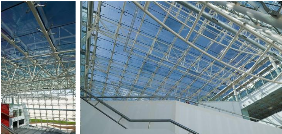
FIGURE 2.18: ROOF OF THE WÜRTH LA RIOJA MUSEUM IN AGONCILLO, LA RIOJA (SPAIN), EACH GLASS PANEL IS SUPPORTED BY FOUR ADHESIVE POINT-FIXINGS (PHOTOS COURTESY OF BELLAPART)
