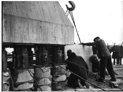
Fig. 5. Jacking up of the towers and positioning of the supporting concrete block.
