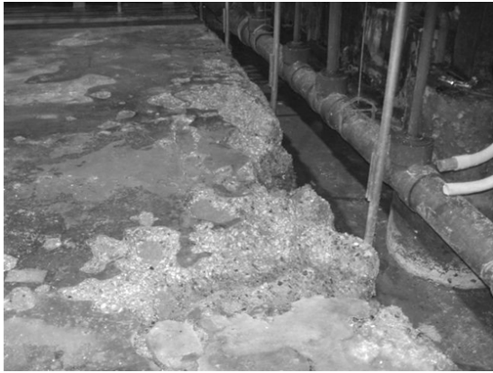
Figure 1: Damage on concrete flooring in a chemical etching plant. The floor was exposed to acid drips and spills. Reproduced from [3] with permission from NACE International, Houston, TX. All rights reserved. ©NACE International 2016.
