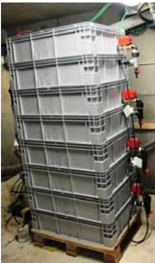
Figure: Greywater treatment plant tower
