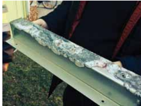
Figure 6: The zinc covering of the steel profile is corroded as a result of direct contact with salty sweat or 'tear' drops from the adjacent MgO-board.
