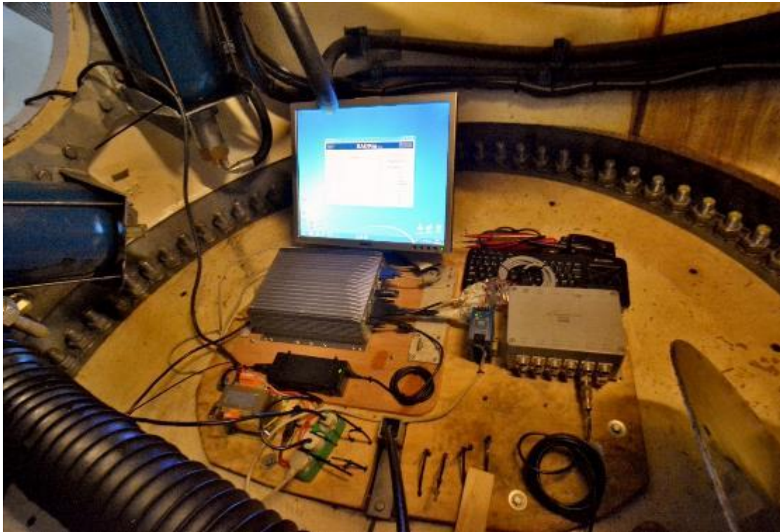
Figure 29. Data acquisition unit installed inside the hub.
