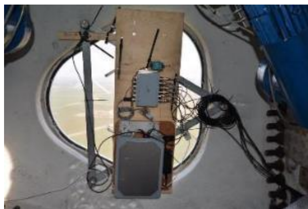
Figure 39. Data acquisition unit installed inside the hub.
