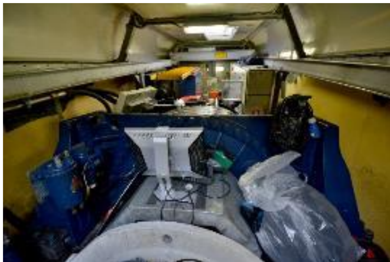
Figure 23. Working area in the nacelle.
