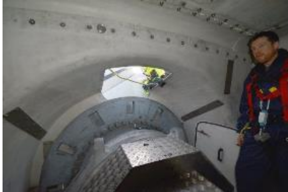
Figure 33. entrance hole to the hub from the nacelle.
