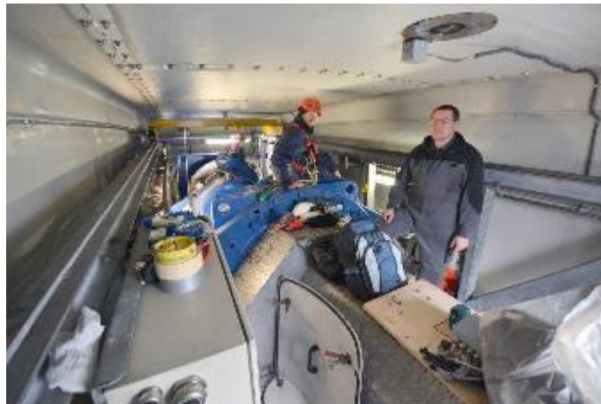
Figure 32. Working area in the nacelle
