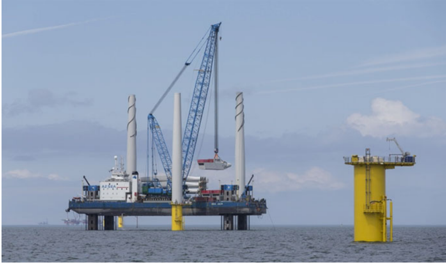
Fig. 19.1 A2SEAs SEA JACK during the construction of the Gwynt y Mor wind farm. Image Source: A2SEA (2016)
