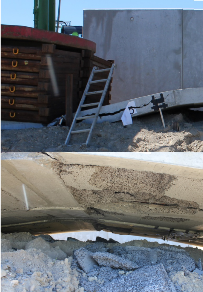
Figure 20: Photographs taken after collapse: longitudinal crack at 3/8 point (top) and crushed concrete at 5/8 point (bottom).
