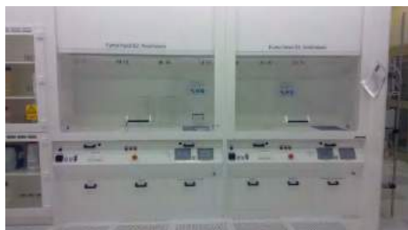
Figure 1: A row of newly installed fume hoods at DTU Danchip. All are equipped with energy saving.
