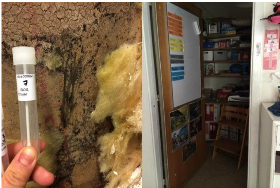
Fig. 22 The case of water-damaged kindergarten presented in Paper 5: to the left gypsum wallboard contaminated with Stachybotrys spp., to the right one of the adjacent rooms where sampling of dust took place
