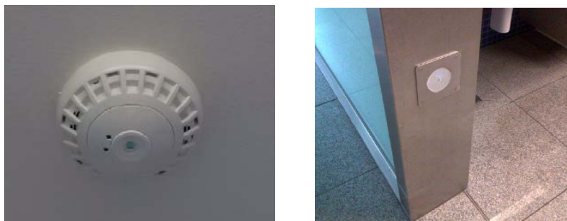
Figure 56. Sensors detecting people entering the room Left photo: Thermal sensor above door. Right photo: Light sensor in door opening. From Paper 6, Fig 8.
