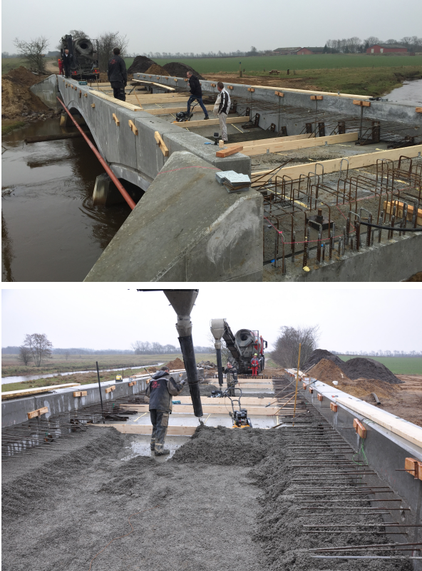
Fig. 1 PCPC cast as fill material in the very first Pearl-Chain Bridge constructed in Denmark in 2015. Upper: The longitudinal bridge section shows that the bridge consisted of a main arch between two adjacent half arches. Lower: Placement of PCPC fill. The formwork wood beams were removed as the different layers were cast.
