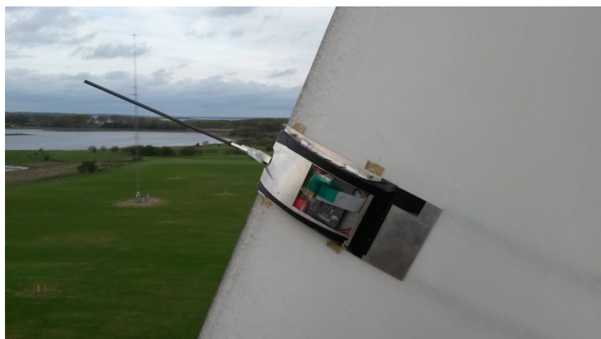
Figure 146 Pitot view from front of the turbine
