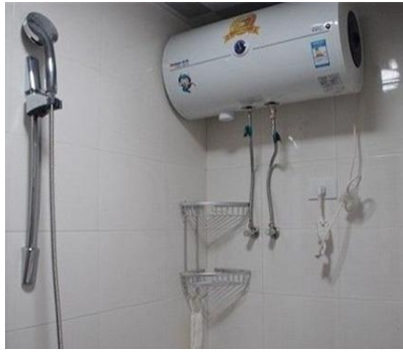
(a). Electric water heaters
