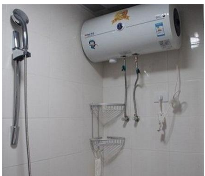
(a). Electric water heater
