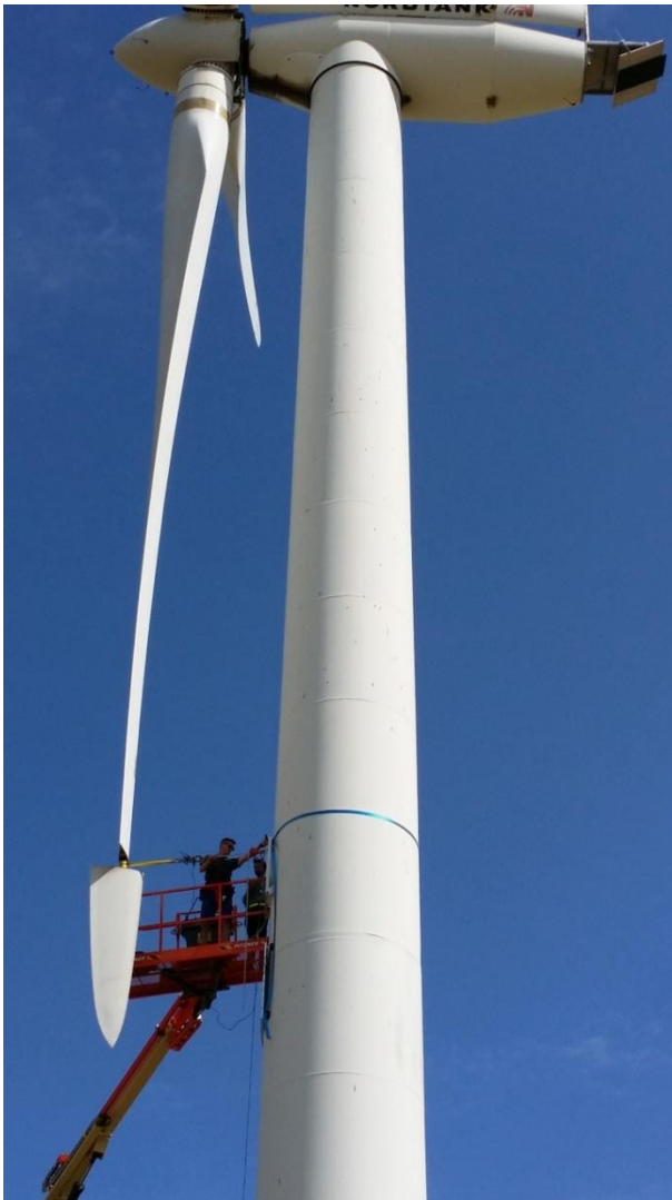
Figure 15 Picture of one of the blade being attached to the tower for the flapwise bending moment strain gauge calibration
