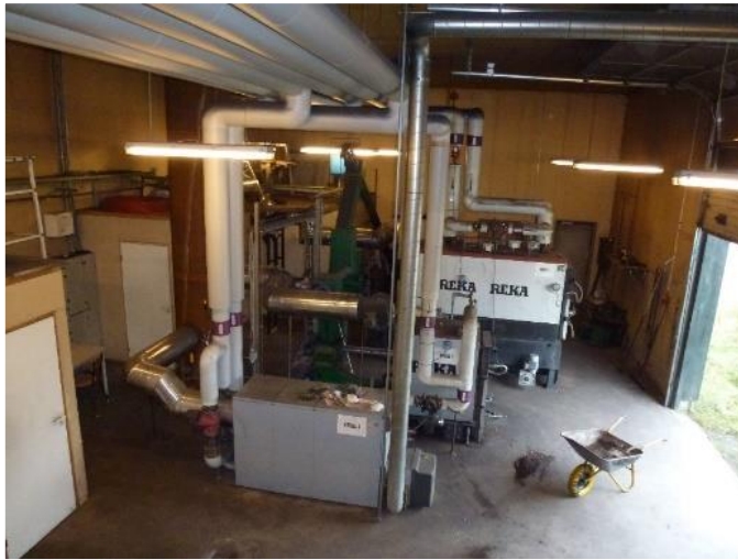
Figure 11. The three existing boilers - 250kW oil boiler (in front), 60kW wood pellet boiler (in the middle) and the 200kW wood pellet boiler (in the back)
