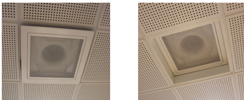
Fig. 2 Fan coil position in baseline condition (left) and in diffuse ventilation condition (right)
