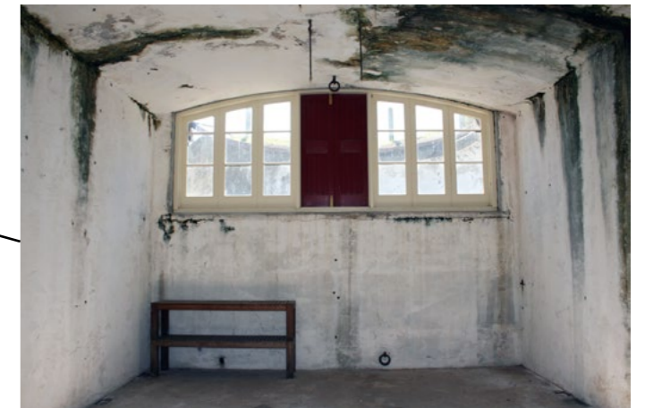
Magazine between gunpits 1 and 2, one of the original 1880 rooms in the fort. The loading galleries are located behind. UQ, 2016
