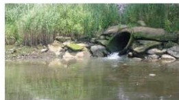
Storm drain outfall at Moody Lane. Photo: Earthplace.
