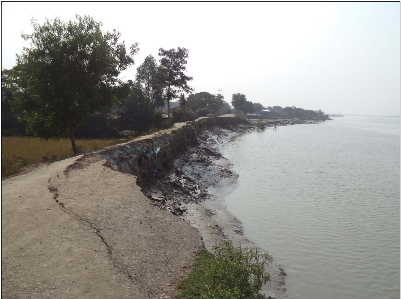
Figure 3.6 Embankment erosion in Laxmikhola in 2013
