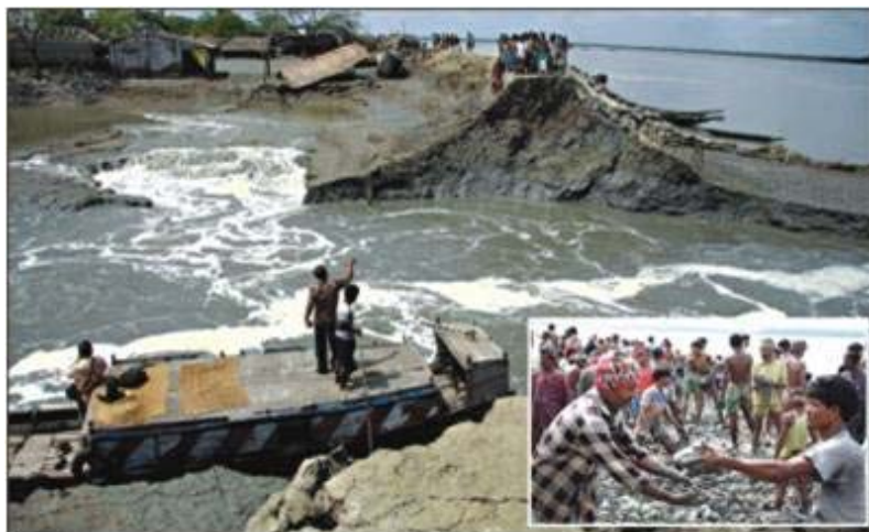
Figure 5.4. Embankment breach during cyclone Aila, 2009; inset - repairing embankment collectively (Source: The Daily Star , 31 May 2009)
