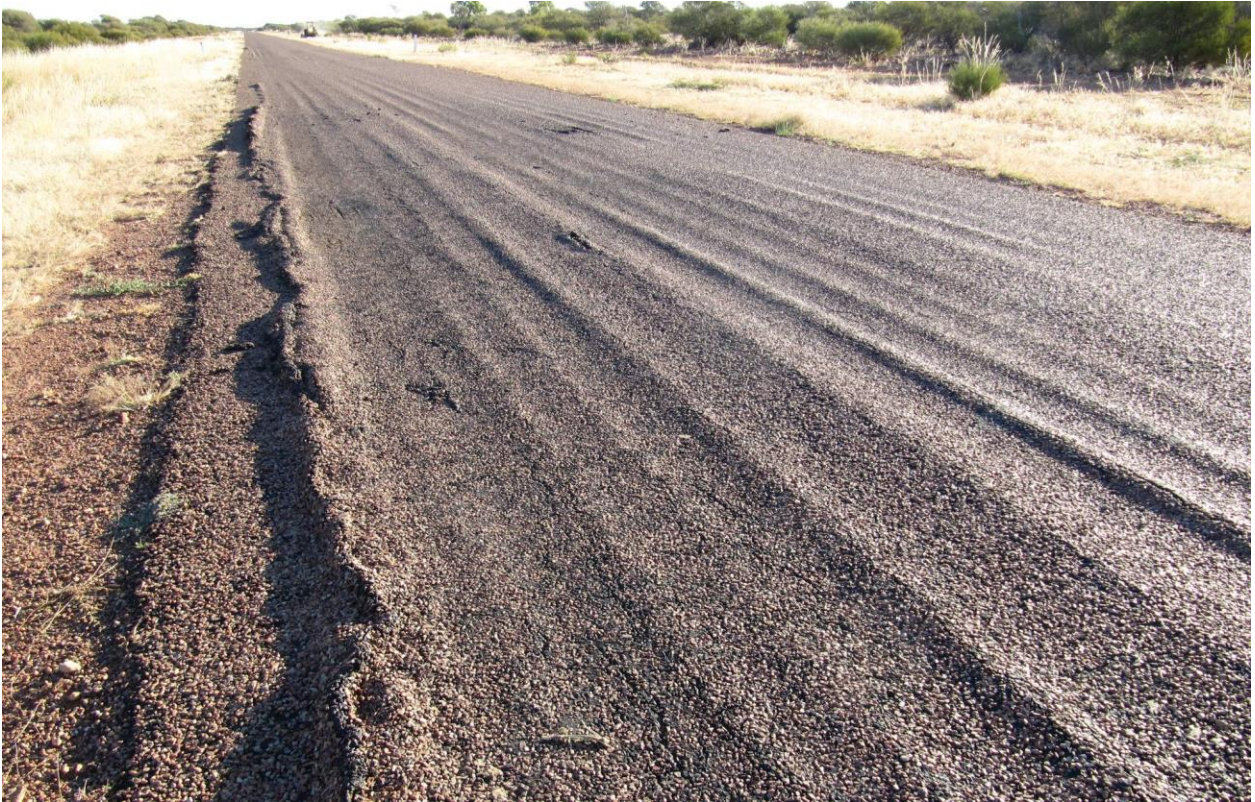
Figure 1-1: Heavy vehicle damage of a flood-affected UBG pavement on the Thompson Developmental road, Queensland, May 2011 (Photo credit: Steve Hogan, Department of Transport and Main Roads)
