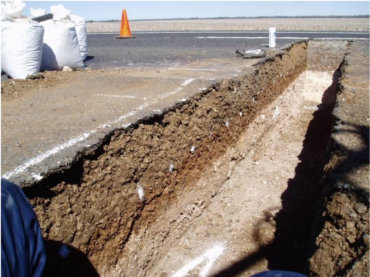
Figure 2-1: A typical thin bituminous pavement with UBG layers (Photo credit: Dave Christian, Department of Transport and Main Roads)
