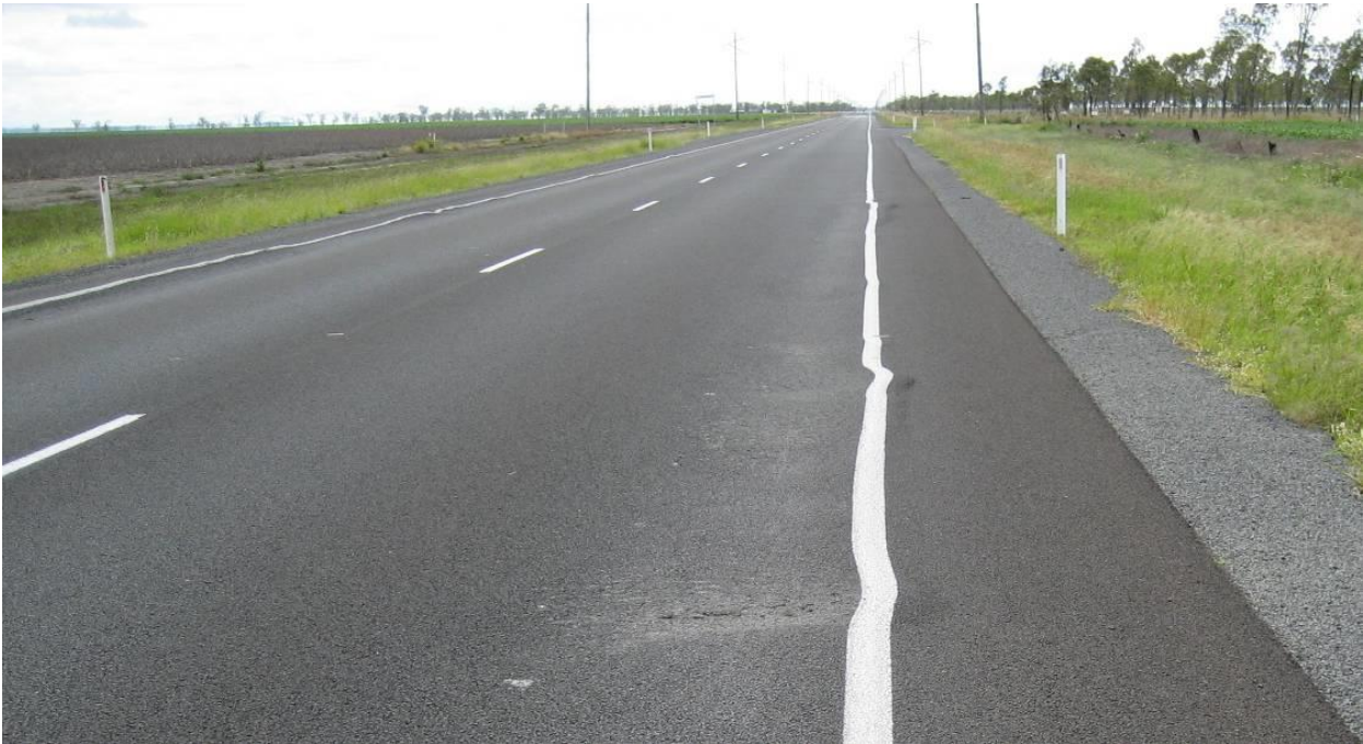
Figure 1-2: Early pavement failure due to excessive moisture and elevated DOS conditions within UBG layers of a recently rehabilitated pavement. Warrego Highway near Dalby, Queensland (Photo credit: Dave Christian, Department of Transport and Main Roads)
