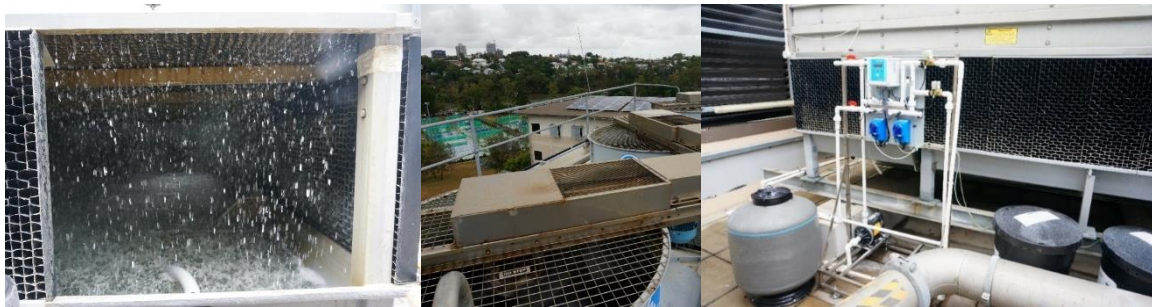
FIGURE 2.8:COOLING TOWER PHOTOS
