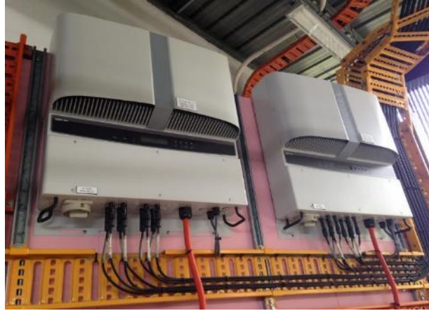
Figure 5.7. Grid Connected Three-phase PV Inverters at UQ PV Site.
