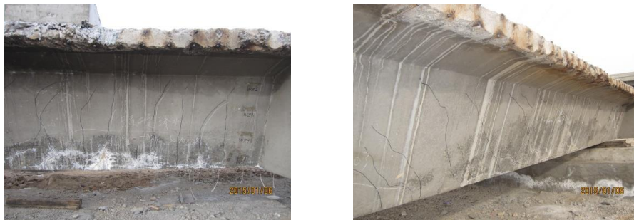
(a) Vertical cracks near mid-span region (b) Inclined cracks outside of pure bending region Figure 3 Failure mode of full scale test girder without strengthening
