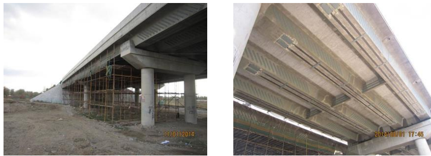
(a) Right half of bridge (b) Strengthening at bottom plate and web Figure 12 In-situ bridge after strengthening
