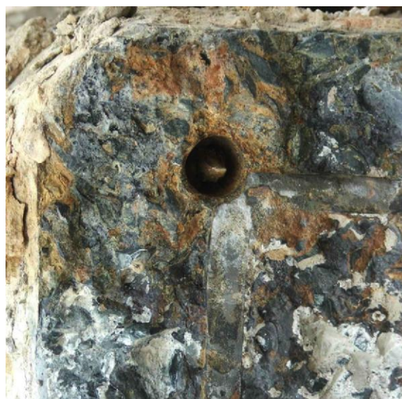
Figure 4 Close-up of reinforcing bar at top left of Figure 3 showing extensive inwards corrosion. (Photo courtesy of Clayton Smith).
