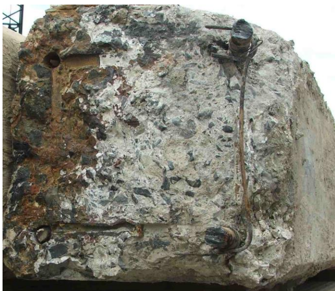
Figure 3 Cross-section of cracked pile showing rust-stained cracking (left) and flame cut bars and freshly broken concrete (right). (Photo courtesy of Clayton Smith).
