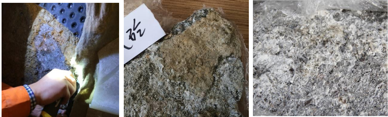
Figure 2 Deteriorated concrete behind the waterproofing board and a white substance on surface
