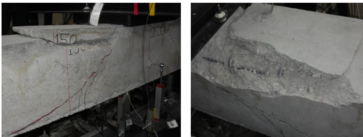
Figure 5 Concrete cover disintegration and concrete crushing at the top next to the contact surface
