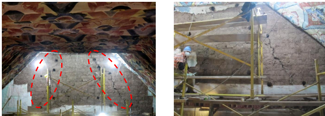
Figure 3 Deep fissures on the triumphal arch of Andahuaylillas church
