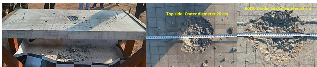
Figure 4 NRC slab under 0.1 kg TNT contact explosion
