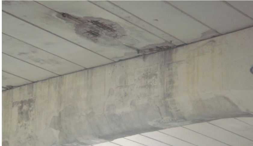
Figure 1 Damage to bridge structures observed in 2010 in Toronto, Canada, due to corrosion of steel reinforcement
