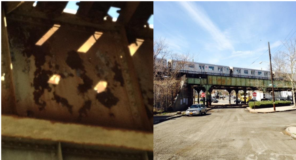
Figure 1 Corroded railway plate girder Bronx-Edenwald, USA.
