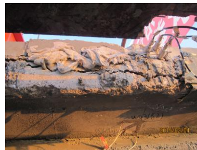
(b) Diagonal crack of top flange in SPCCS-S-1
