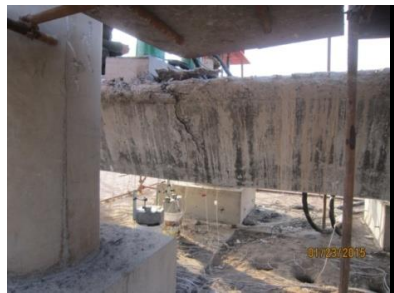
(a) Web cracks of N-S-1
