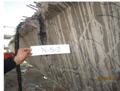
(b) Web cracks of N-S-2
