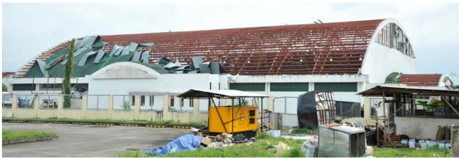
(a) Damage to roof cladding materials of EGS Contact Center
