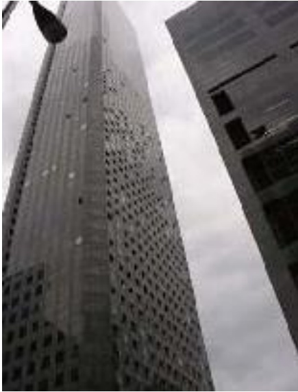
(a) Damage to window panes
