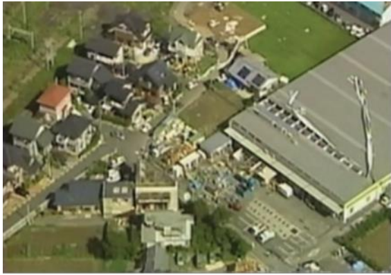
(a) Partial damage to metal roof sheets
