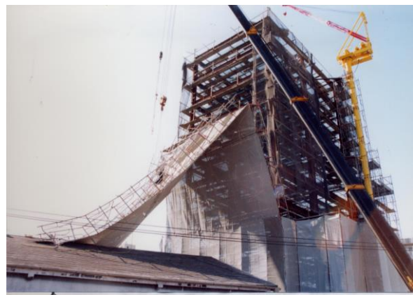
(b) Damage to scaffolding and induced damage to neighboring buildings (Ohdo, 2007)
