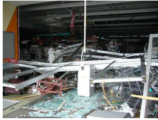
(b) Induced collapse of entrance sashes and doors
