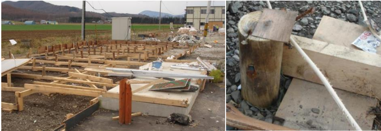
Figure 7 Simple foundation system of construction work offices shown in Figure 6 (Tamura et al. , 2007)
