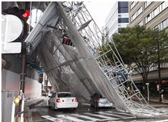
(a) Damage to scaffolding and induced car accidents (Hokkoku Shimbun, 2007)
