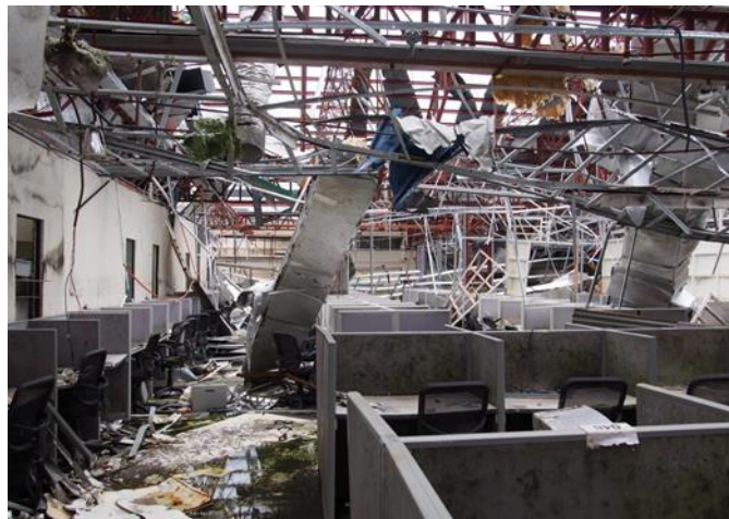
(b) Serious property damage inside and failure of business continuity planning (BCP)
