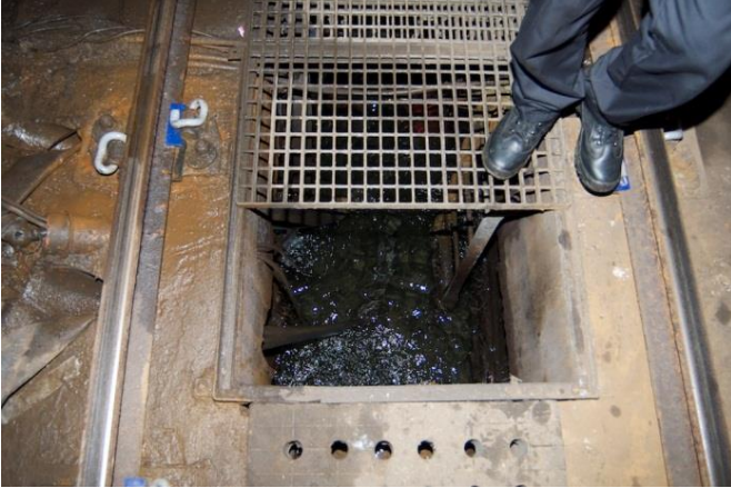
Figure 4: A typical sump located between the rail tracks in the Glasgow Subway system.
