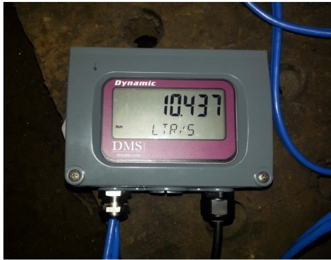
Figure 7: The ultrasonic flow meter showing the water flux (l/s)
