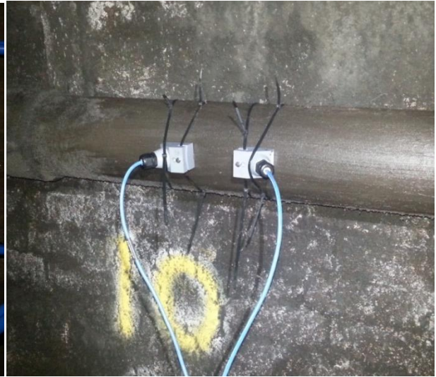
Figure 8: The transducers clamped onto the discharge pipe
