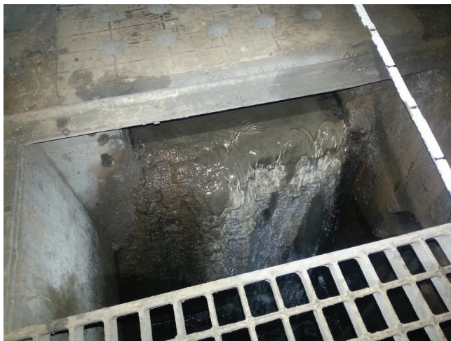
Figure 3. A typical sump located between the rail tracks in the Glasgow Subway system
