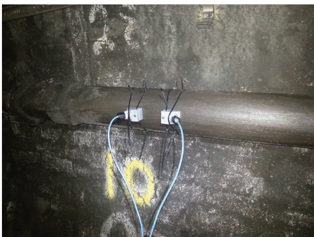
Figure 5. The transducers clamped onto the discharge pipe
