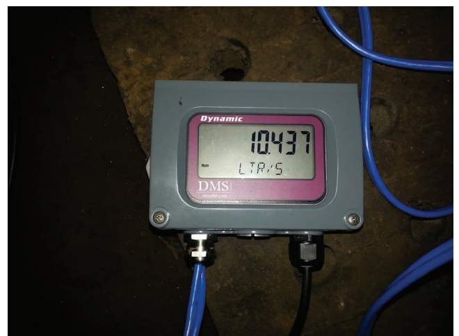
Figure 6. The ultrasonic flow meter showing the water flux (l/s)
