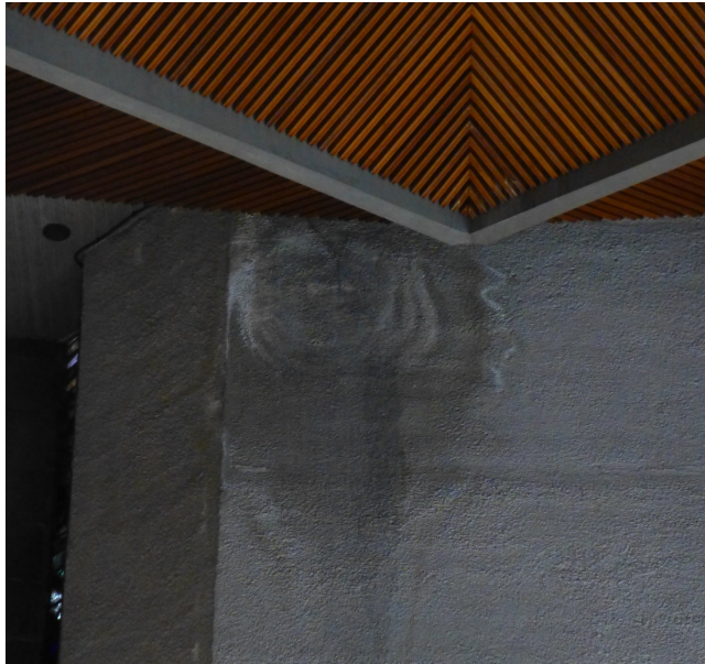
(b) Internal water staining
