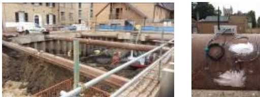
Figure 7. Field deployment of the wireless strain sensor network at the Trinity Hall excavation site.
