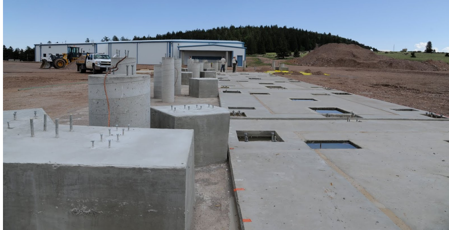
Figure 3: The first three foundation pads for unit telescopes on the West arm of the MROI, together with the beam-relay piers. A total of seven foundation pads have been constructed so far. The MROI beam combining facility is in the background.
