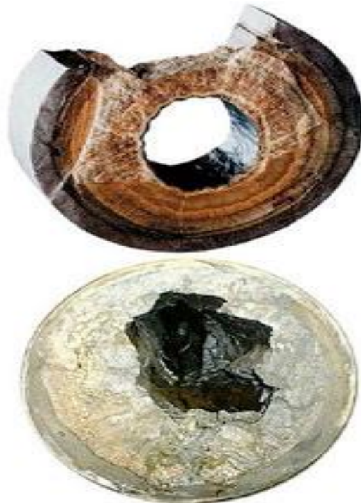
Figure 2-1. Image of scale deposition in a pipe [9]
